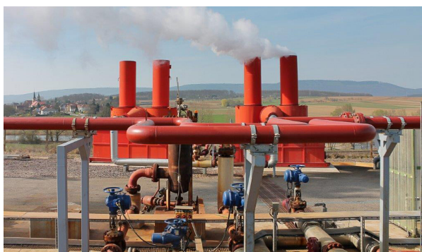
Geothermal power plant in Souz.
