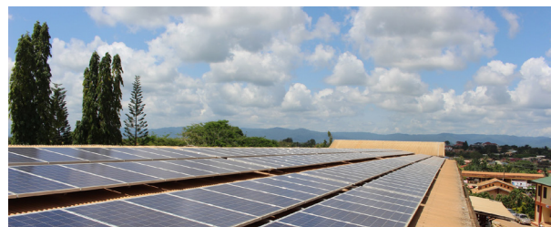
Installed PV modules, St. Dominic’s Hospital Akwatia, Ghana.
